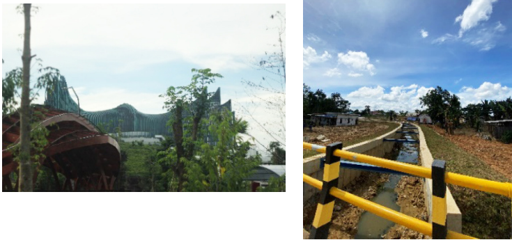
Figure 22 KIPP and Flood Control Construction Project in Bumi Harapan Village (Source: Authors, 2025)
